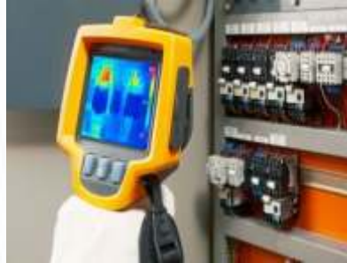
THERMOGRAPHY OF LT PANEL
